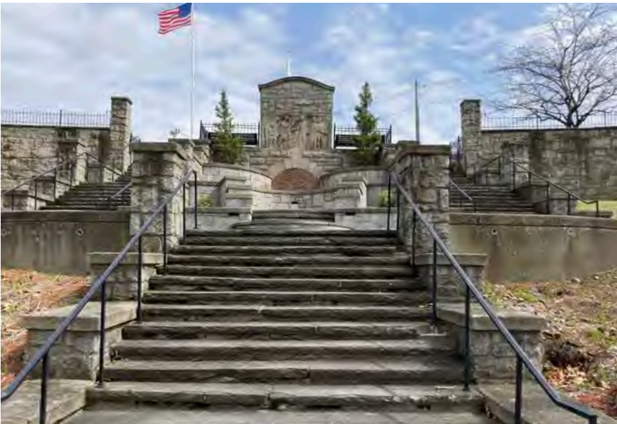
Sweatt Park is a attractive location in Wrentham Center that remains difficult to access for the handicapped, elderly and families with strollers. An ADA assessment would make the Town eligible for funds to provide better access to this and other locations.
